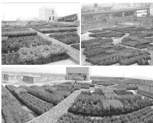
Figure 4 Sustainable extensive green roof at Delta Electronics Inc., Tainan Plant, Taiwan. Photograph credit: Yu-Wei Ho
